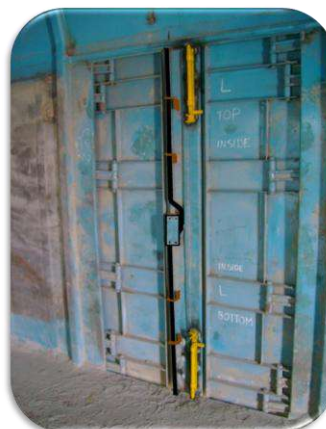
Inner view of additional door locking arrangement
