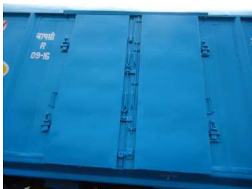
Outer view of door locking arrangement
